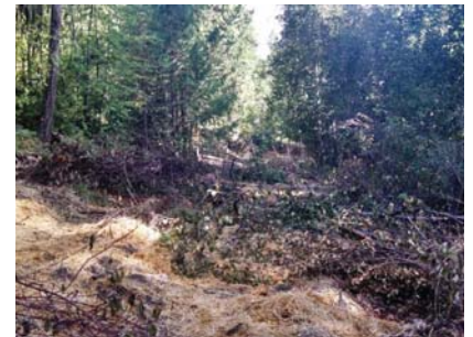
The water is put back into its original bed, and the old road is reclaimed as a riparian buffer.
